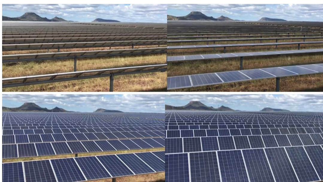
Plate 2-4: East-West Single Axis Tracker System, Finished Array
